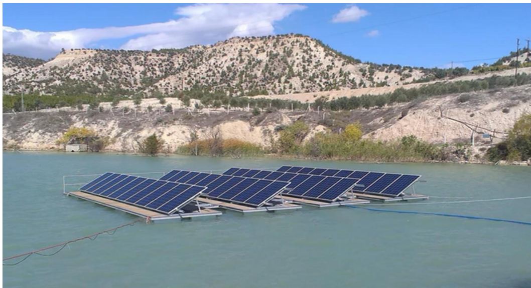
Figure 2.6 FPV installation in Azmak 2 HEPP, Mersin (Bulut et al., 2018)
